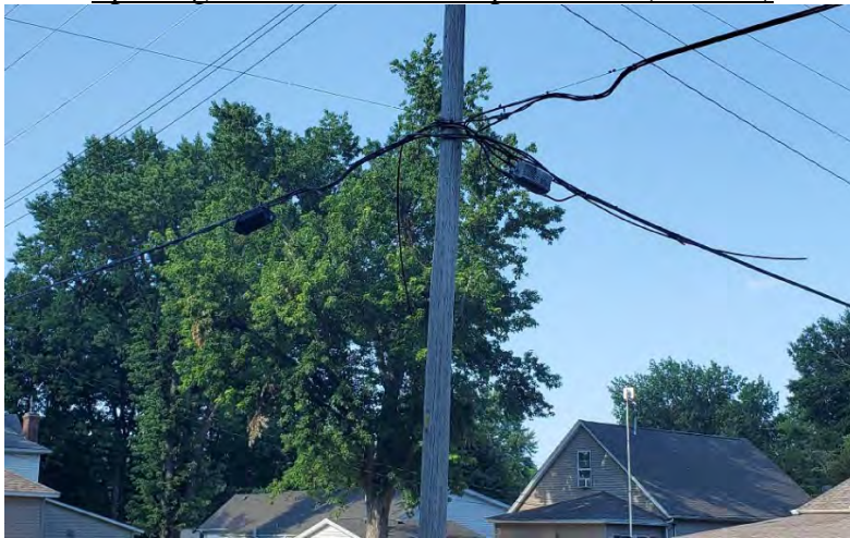
Sparklight Fiber Node and Splice Case (Auburn)
