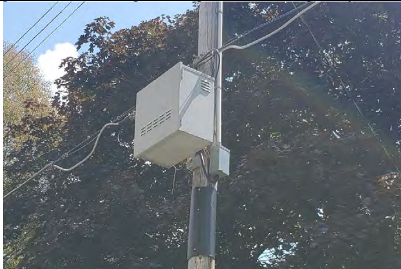
Sparklight power enclosure for power/amplification and capability for battery backup
