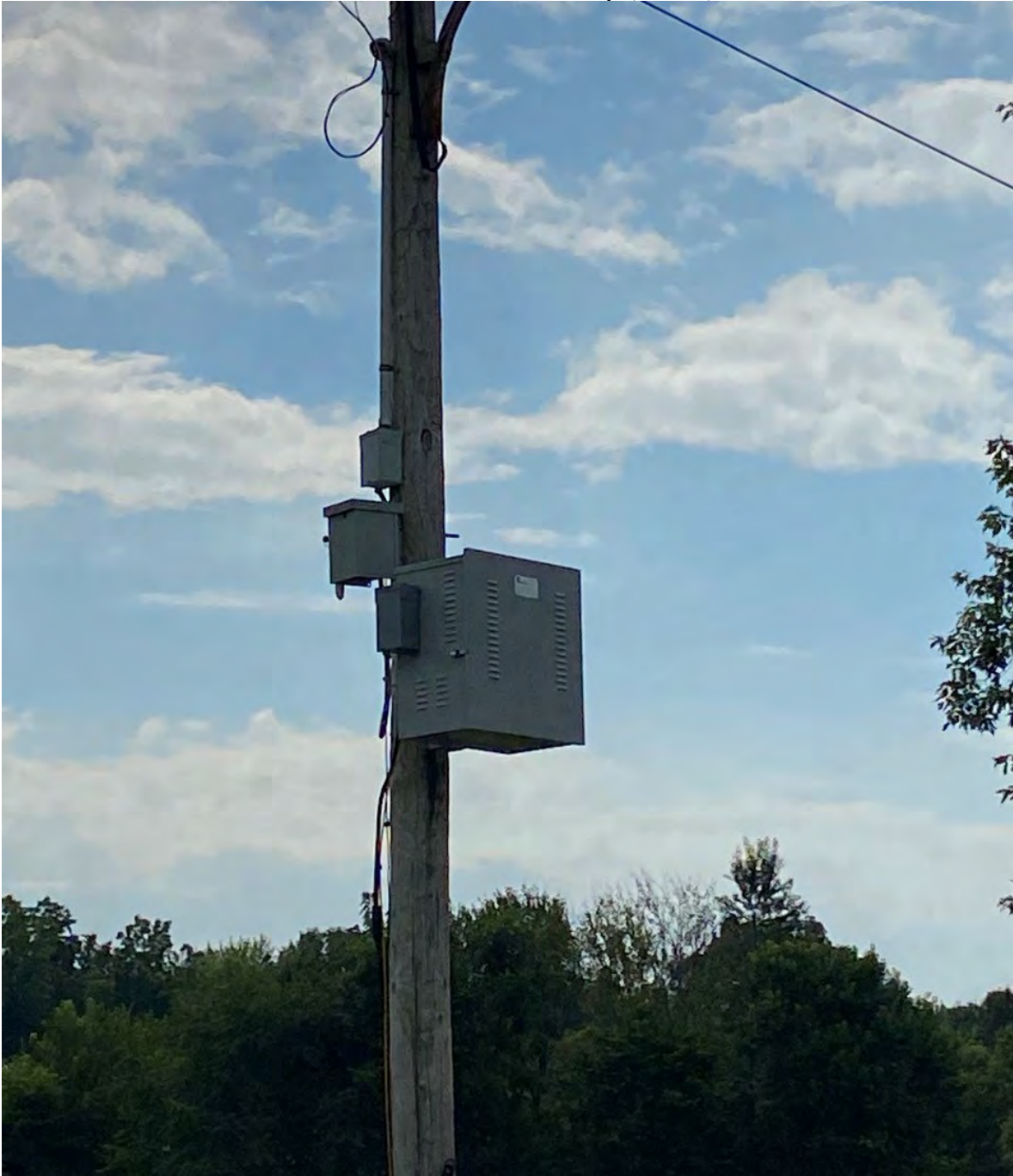
Mediacom Cable Power amp (Loami)
