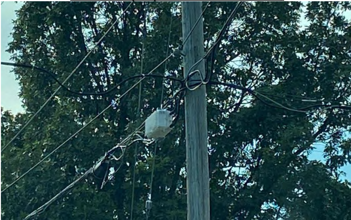
Comcast fiber splice point and cable node (Rochester)
