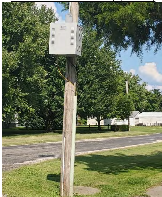
Mediacom Cable Power amp (Dawson)
