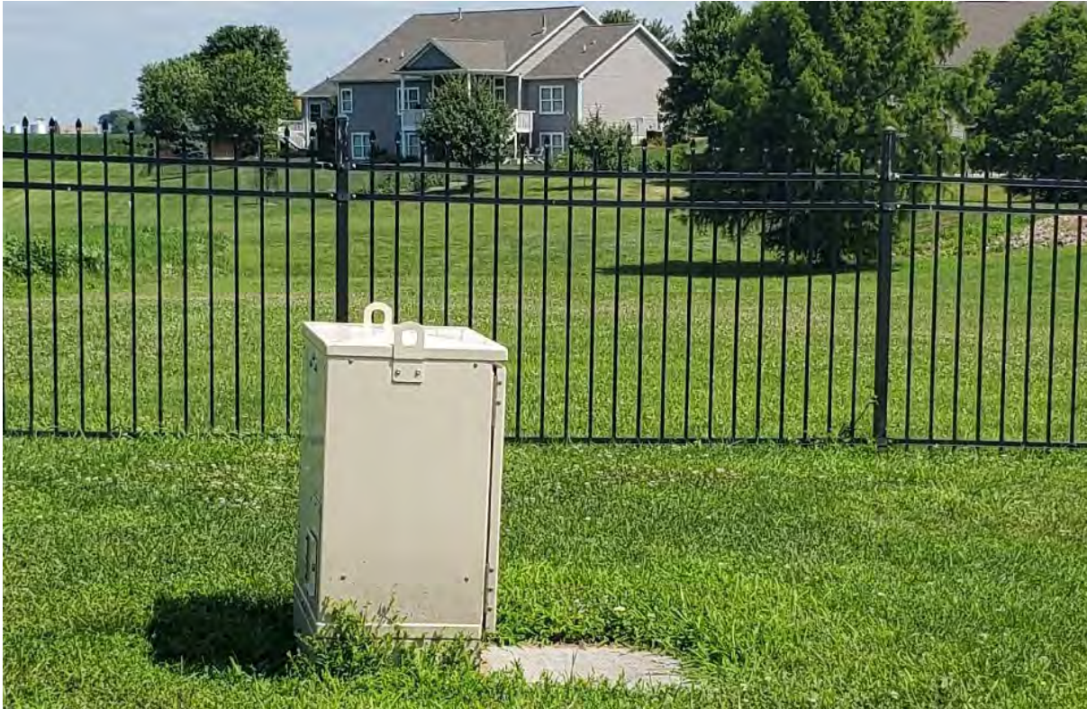
CASSCOMM PON Cabinet at Rail Golf Course (Sherman)
